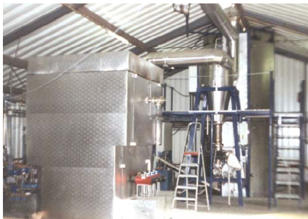
Manure gasification plant in Bladel, the Netherlands
