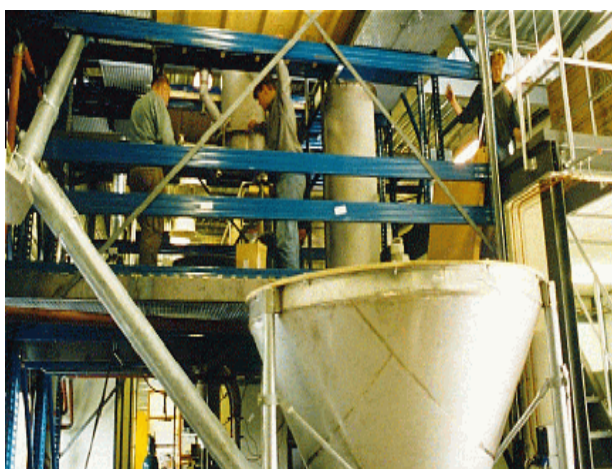
The 5 ton/day pilot plant
